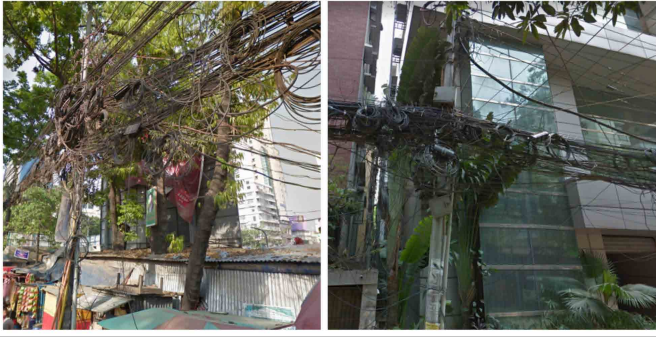
Fig. 5. Images of Wires Collected from Street View
